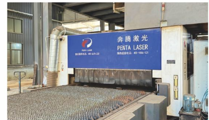
12000W 激光切割区 12000W Laser Cutting Area
