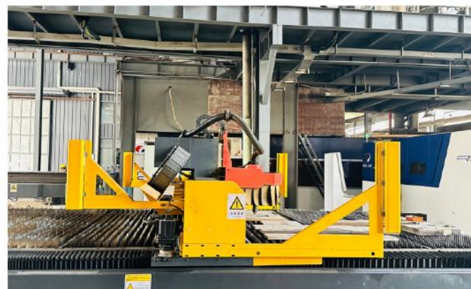
30000W 激光切割区 30000W Laser Cutting Area
