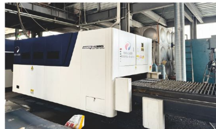
6000W 激光切割区 6000W Laser Cutting Area
